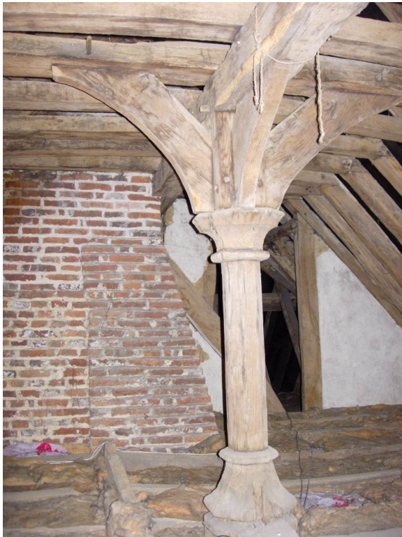
Fig 23 The open-truss crown post at Brewerstreet Farmhouse, Bletchingley , is particularly fine with an octagonal shaft, base and capital. Photograph by Patrick Moyle.
